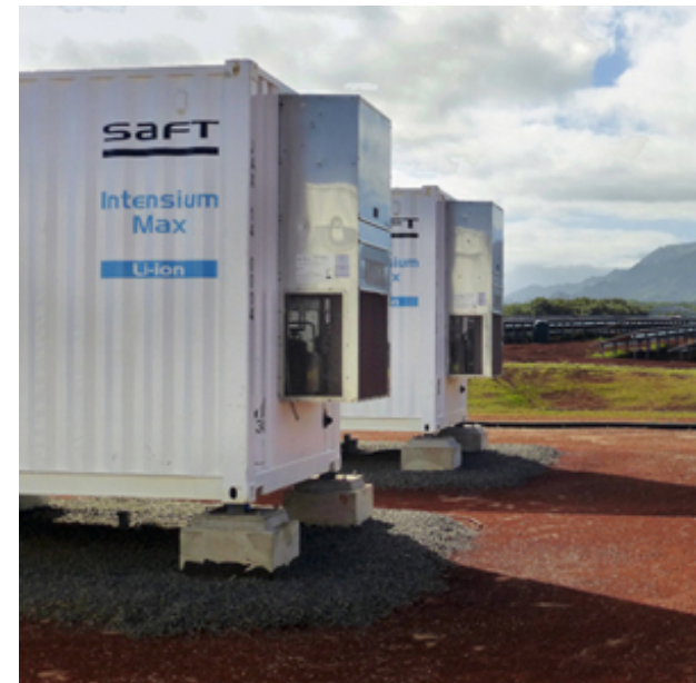
Shipping containers filled with lithium batteries on Kauai, Hawaii USA (Source: Technology Review 2015)
