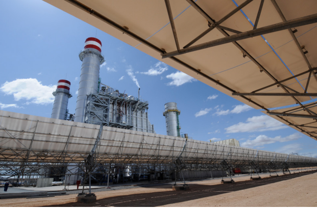
Solar panels at a thermo-solar power plant. © Dana Smillie / World Bank
